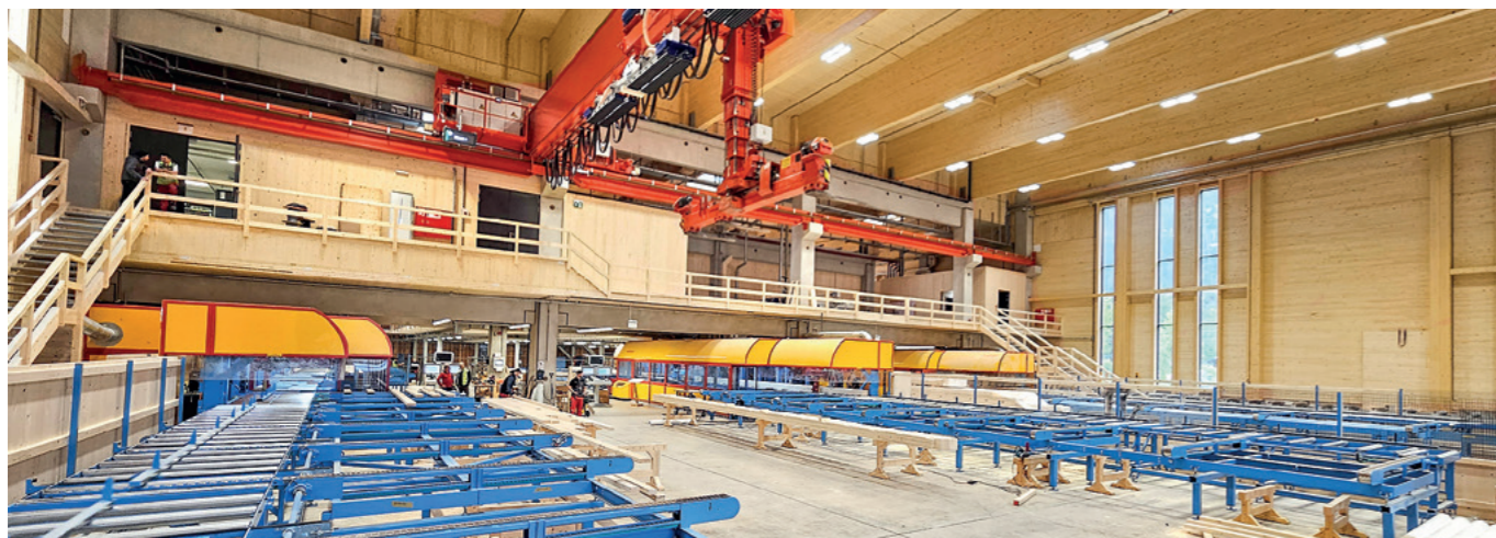
Concentrated joinery performance in Assling: Next to an existing K2i, Theurl had to Hundegger K2-Industry machines installed, thereby bringing its glulam joinery service up to date with the latest technology
